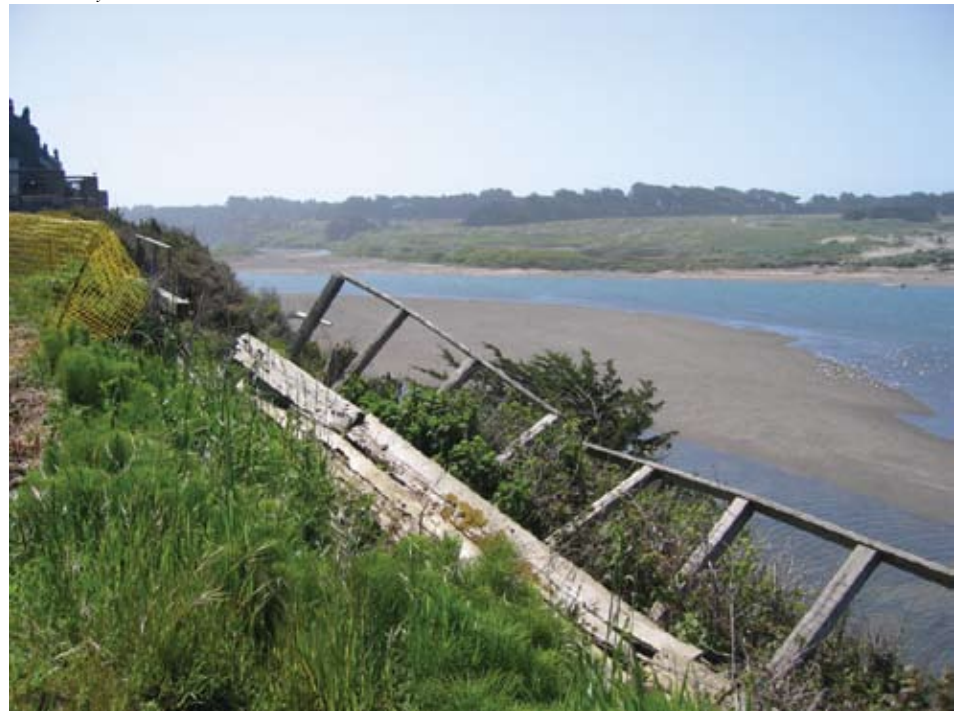
The Coastal Commission has required Mr. Bower to repair this 100 foot retaining wall which failed in February 2006, taking part of the trail easement with it. He has proposed to replace it with a 400-foot-long retaining wall system along the full extent of the bluff face, which he believes will be of greater benefit to his plans for future development.
